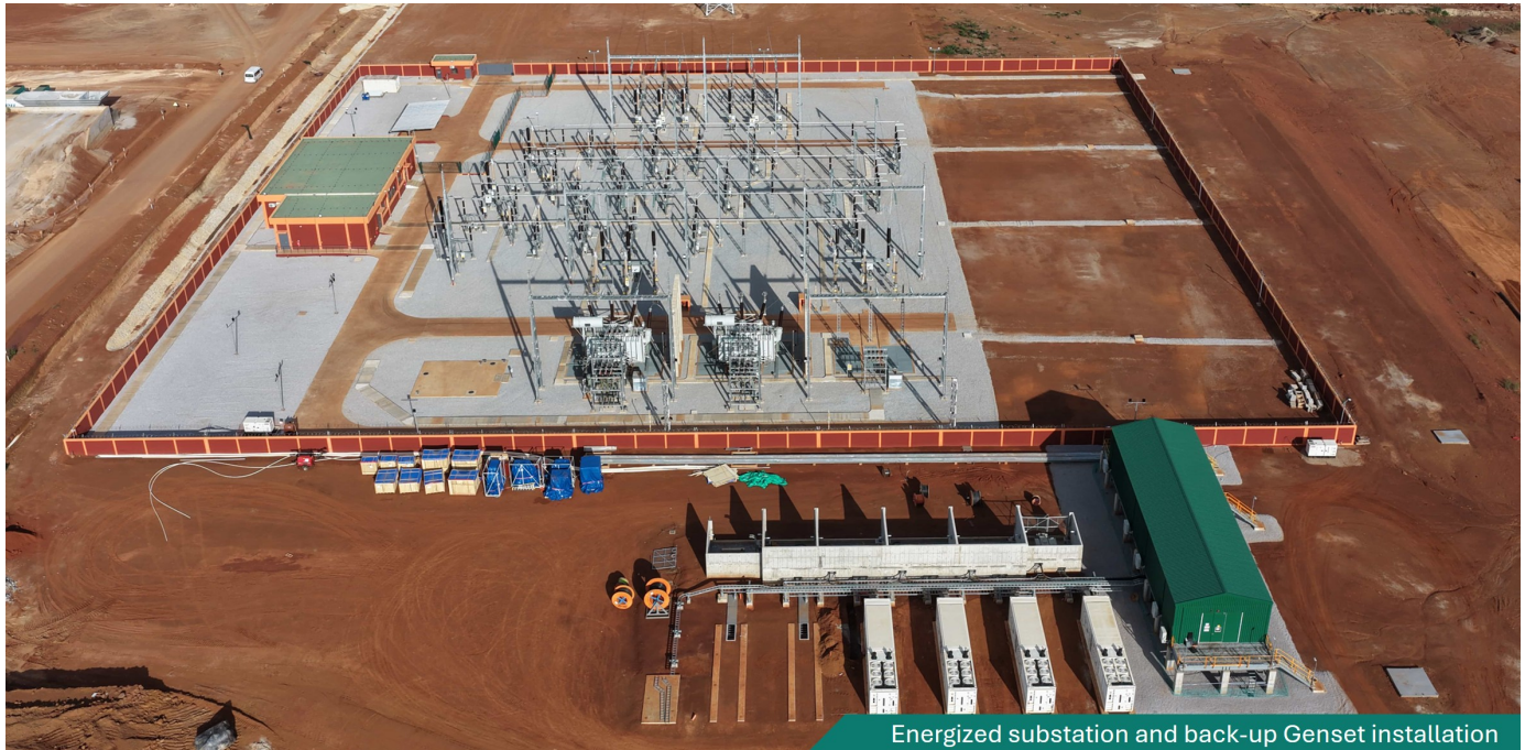
Figure 4: Electrical substation, high-voltage grid connection and gensets
