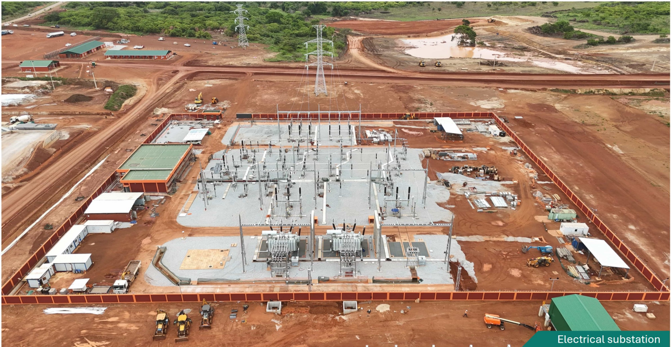
Figure 6: Electrical substation and high-voltage grid connection preparation
